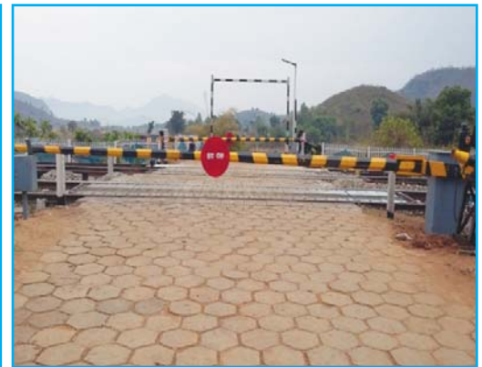
Electric Lifting Barrier
