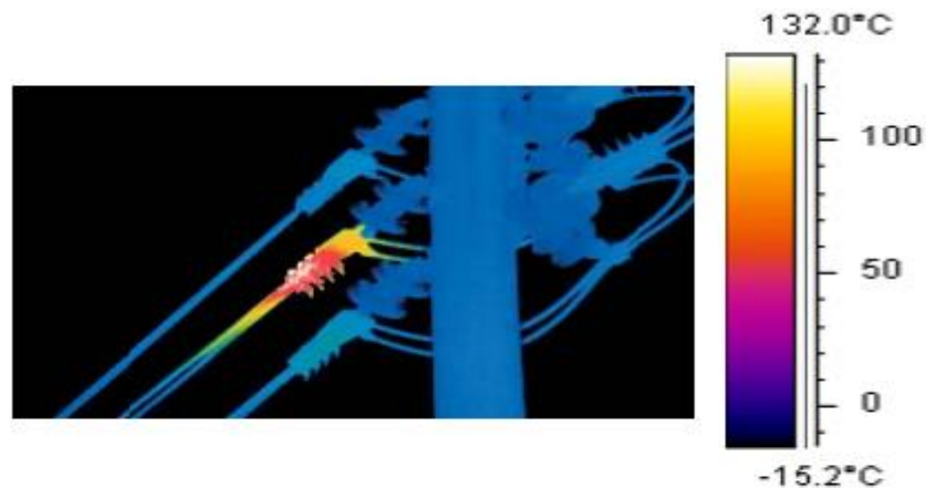
Thermal image showing over heated loose connection with temperature chart
