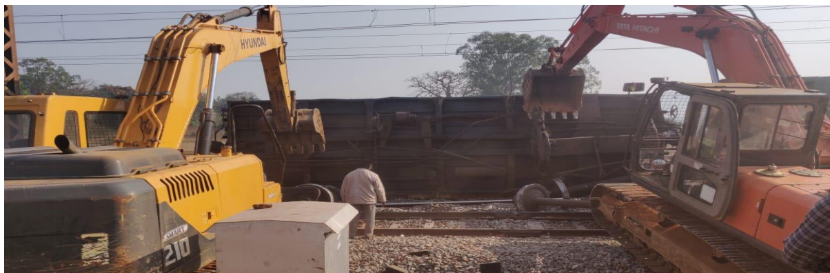
DERAILMENT DUE TO UNEVEN LOADING & RESTORATION WORK
